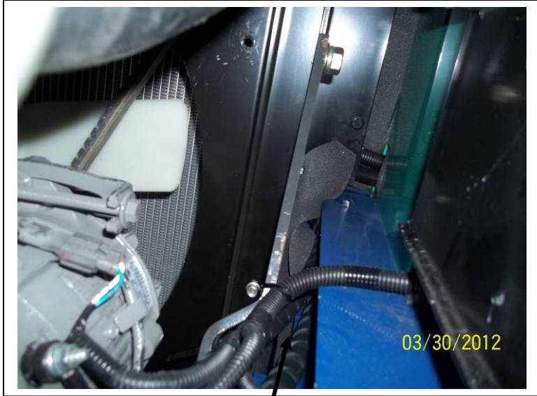
13/32" line going into radiator compartment
