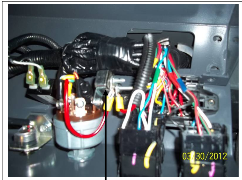
20 amp circuit breaker
