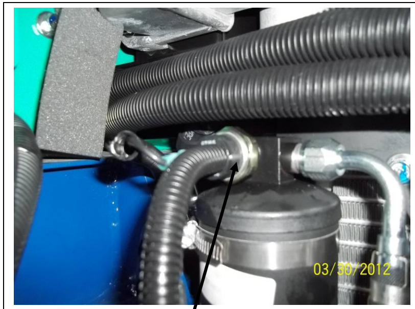
Binary pressure switch mounted on the drier.
